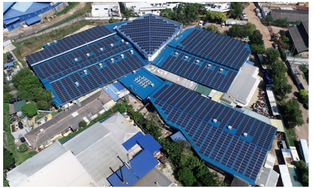
658 kWp Solar Roof Top System, Homagama HI Fashion Holdings (Pvt) Ltd
